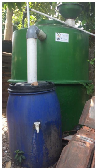
(a) Biodigester (BSO-15)
